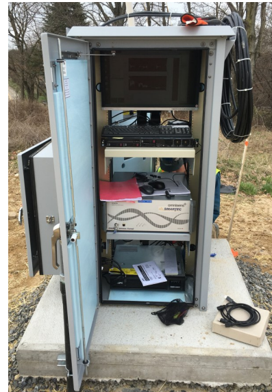
DiTeSt dedicated instrumentation cabinet
