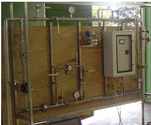
Fig. 14. Gas leakage circuit.
