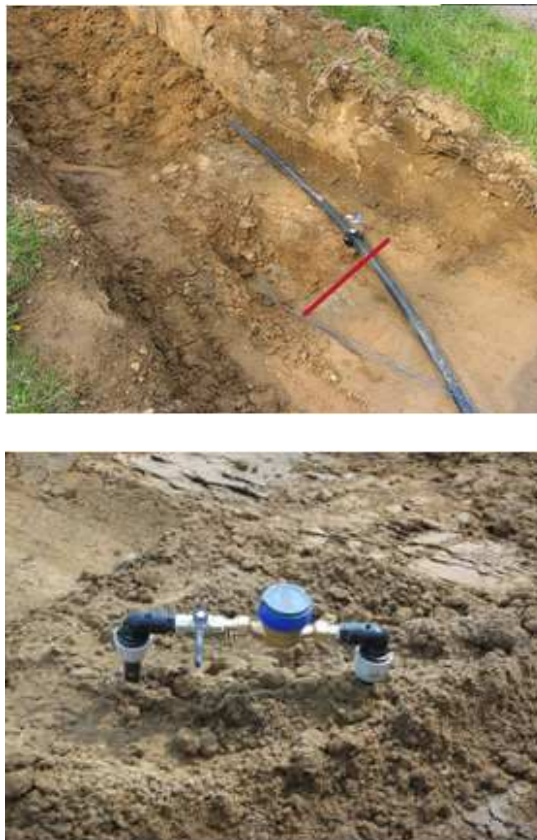
Fig.4. Leakage detection simulation arrangement. Several taps, with volume meters are used to generate controlled leaks.
