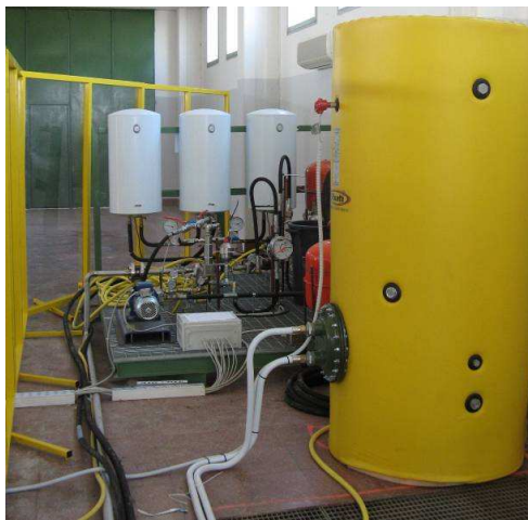
Fig. 12. Liquid leakage circuit.
