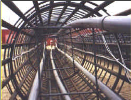
Figure 4. SOFO sensor network (white plastic cables) installed on pile rebars before pouring
