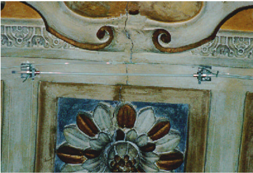
Figure 3: SOFO Sensor Installed on a Church Vault
