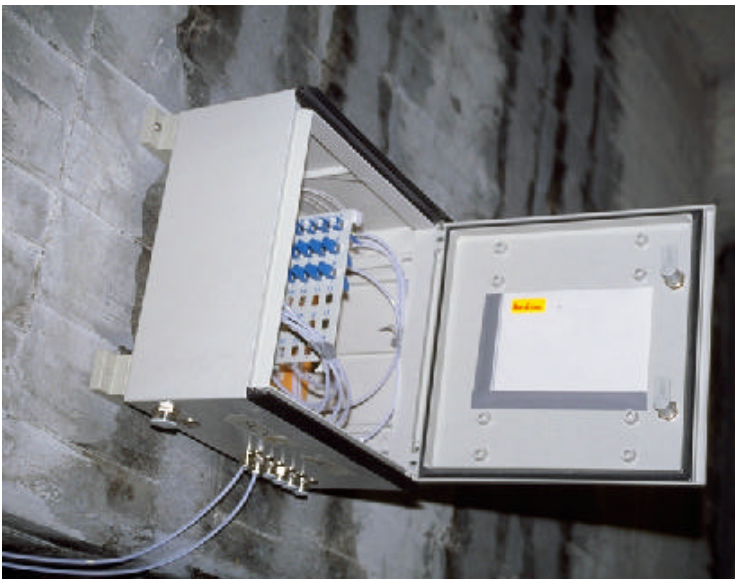
Figure 10: Connection Box for Mating Sensor Cable with Multi-fiber Extension Cables
