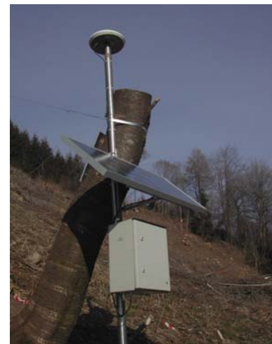
Figure 2: 3DeMoN-GPS rover measurement station with solar power supply
