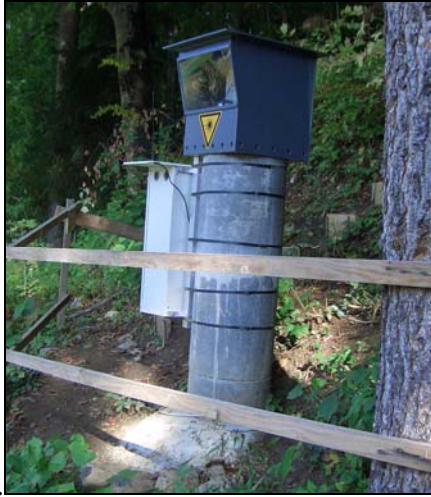
Figure 8: ROBOVEC installed on a pillar
