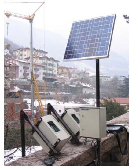
Figure 3: Installation with two 3DeMoN-Laser instruments and a 3DeMoN Monitoring Station with solar power supply
