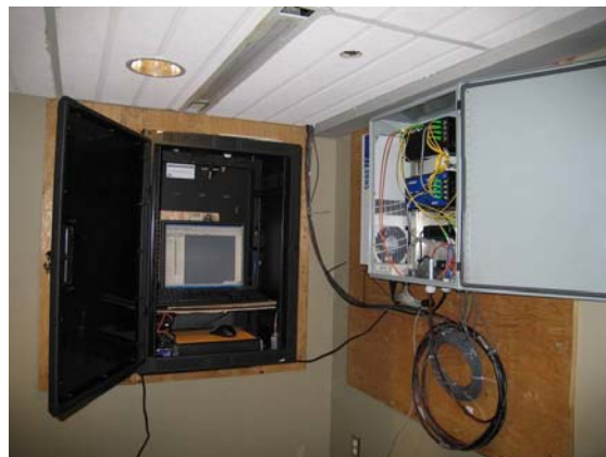
Figure 16: Central Measurement Point with dedicated PC (left) and Fiber Optic reading unit with switch (right)
