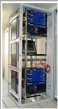
Fully redundant cabinet
